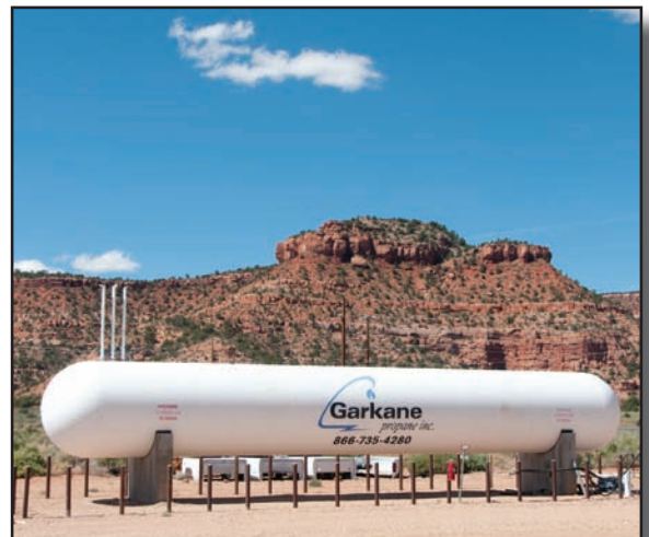
- Propane Storage Tank in Kanab -
